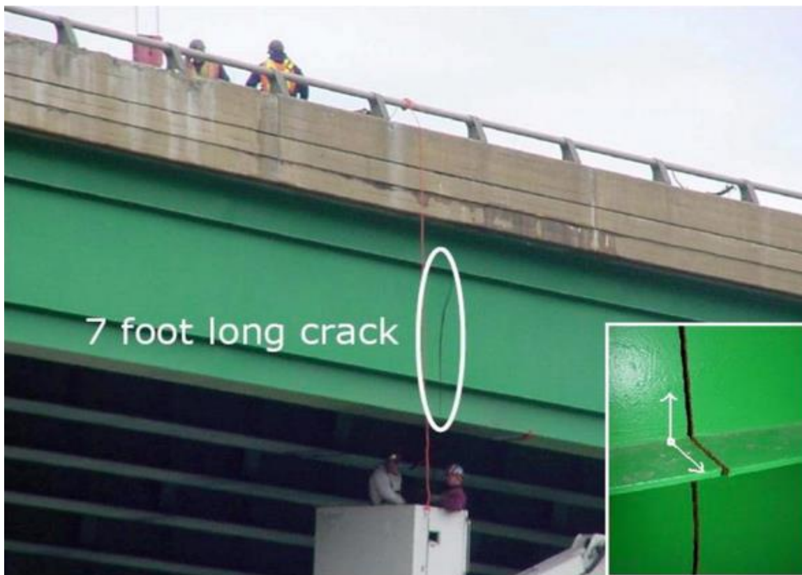
Figure 1-2: Fatigue cracking in a bridge girder from weld defects
